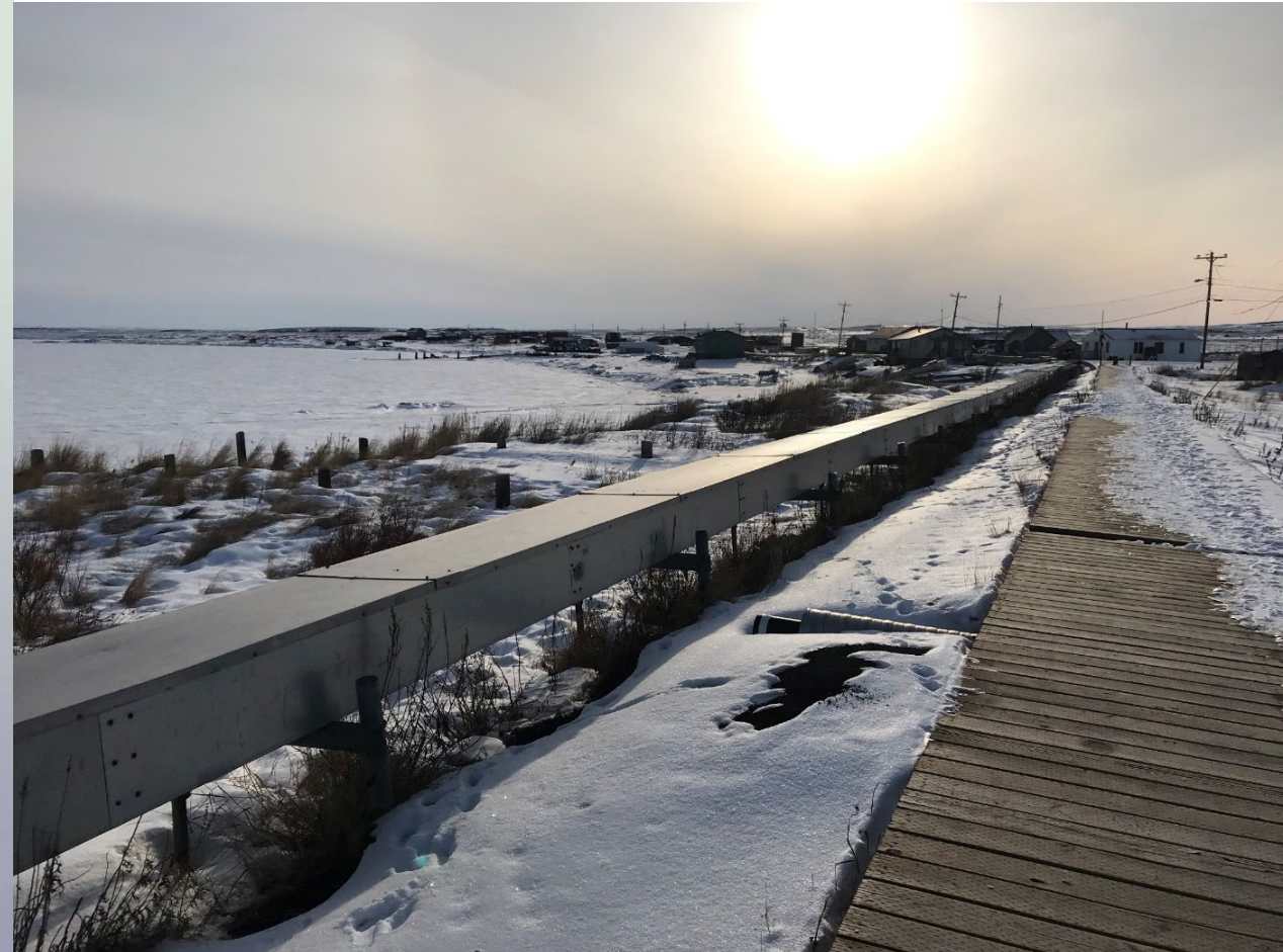
Water and Sewer Utilidor in Saint Michael, Alaska
